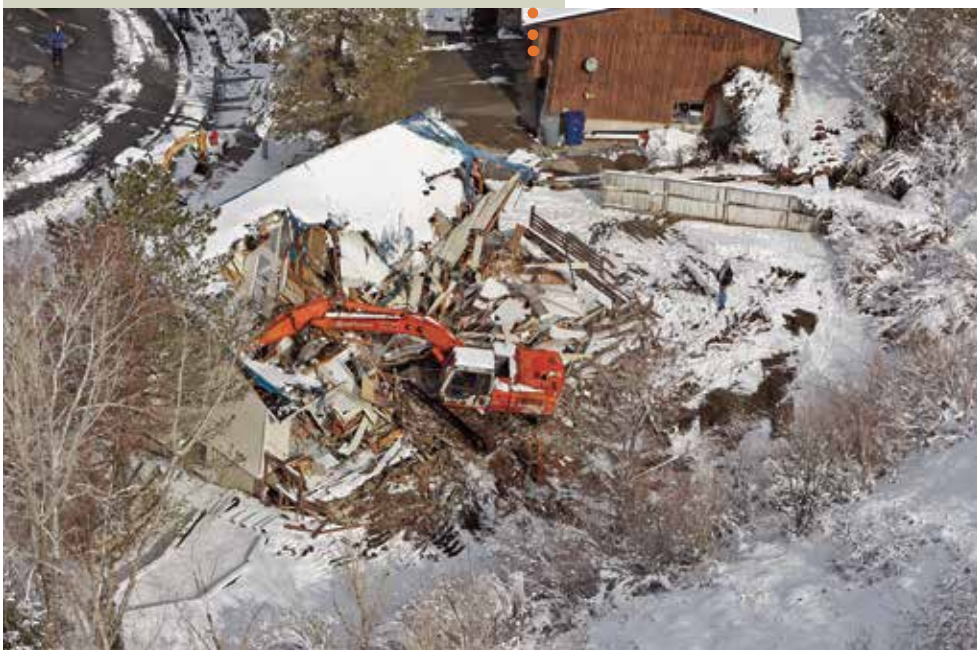
A BACKHOE DEMOLISHES A HOME IN THE PATHWAY OF A LANDSLIDE IN NORTH SALT LAKE CITY, UTAH, 2011.
